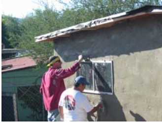
Knox's Ryan Fabrizio and the home owner smoothing the stucco together last year
